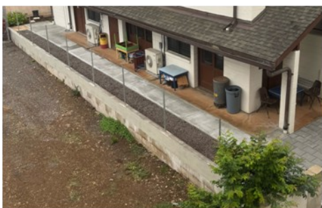
View from above of the repair of the concrete masonry unit fence and sidewalk extension pavers and drainage bed. The panels for the fencing are on order.
